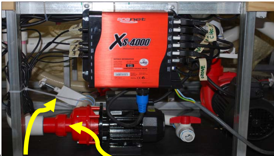
Shut off valve
